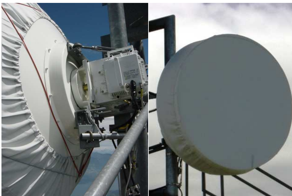
Figure 5 - Teflon cover from Stockhorn 16 months after installation
